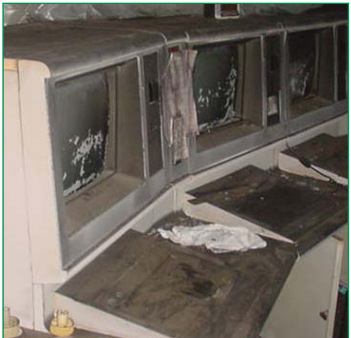
Figure 1. Extensive damage to the control room at IVRR.
