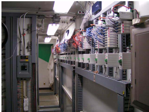
More than 2500 Opto 22 SNAP PAC System I/O points monitor and control water treatment processes around the clock
