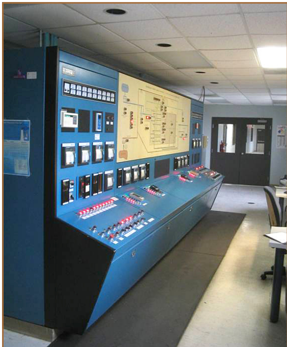
Figure 3. Original analog control system at Otisco Lake Water Treatment Plant, Onondaga County Water Authority.
