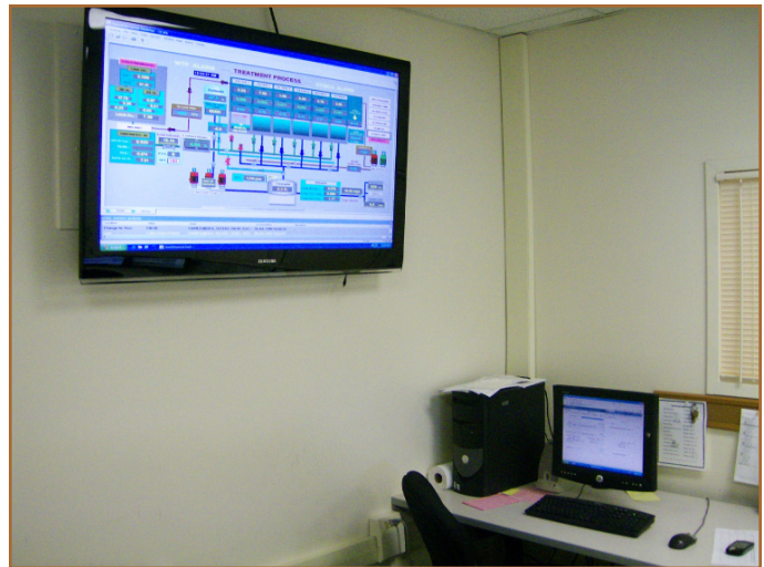
Figure 4. Process functions are now controlled through a PC/PLC-based control system.
